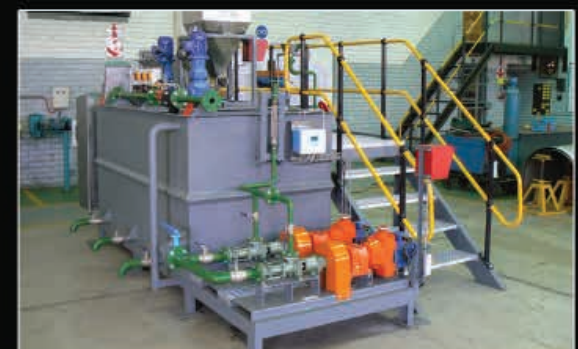
Skid mounted flocculant plant
